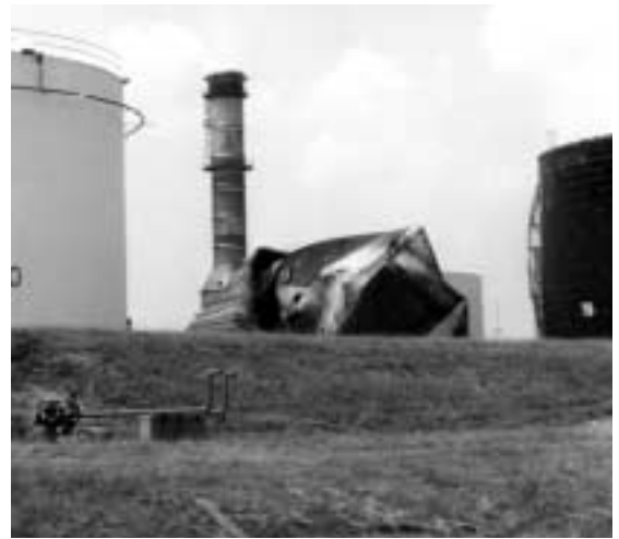
The picture above is not one of the tanks damaged by the explosion. This one, visible from Route 9, collapsed in on itself when an emptying procedure went awry.
